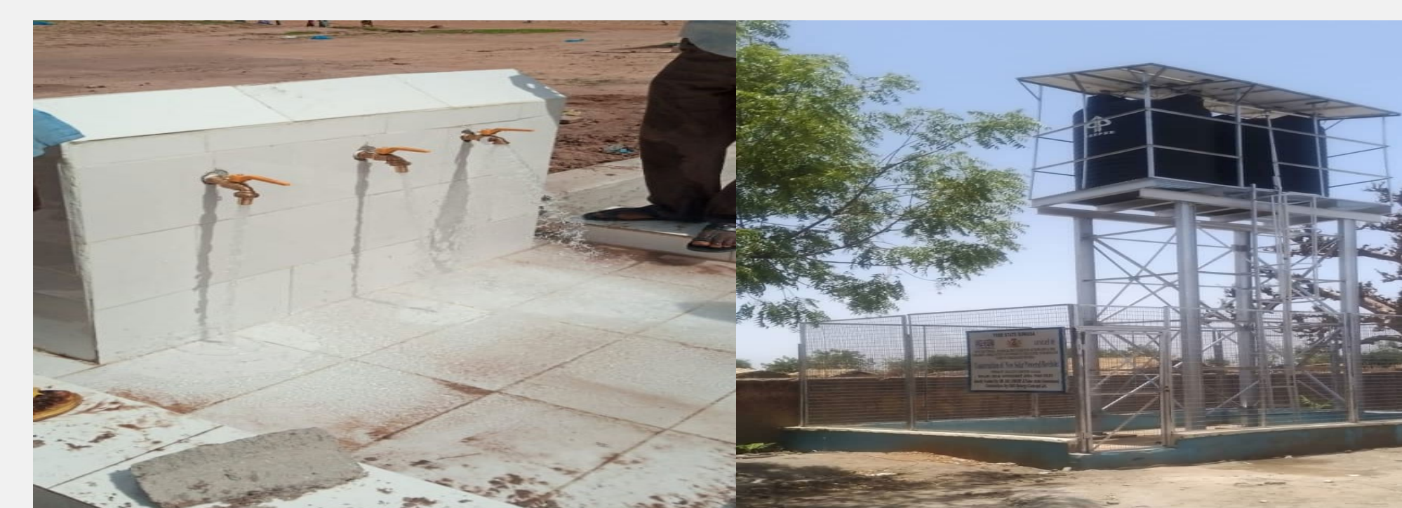
Fig 2 Snapshot of solar newly constructed solar powered borehole in Gabai PHCC of Gulani LGA
