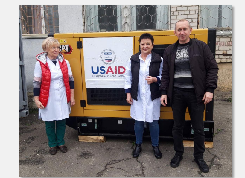
Health workers from Mykolaiv Oblast Hospital stand beside their USAID-distributed generator.
